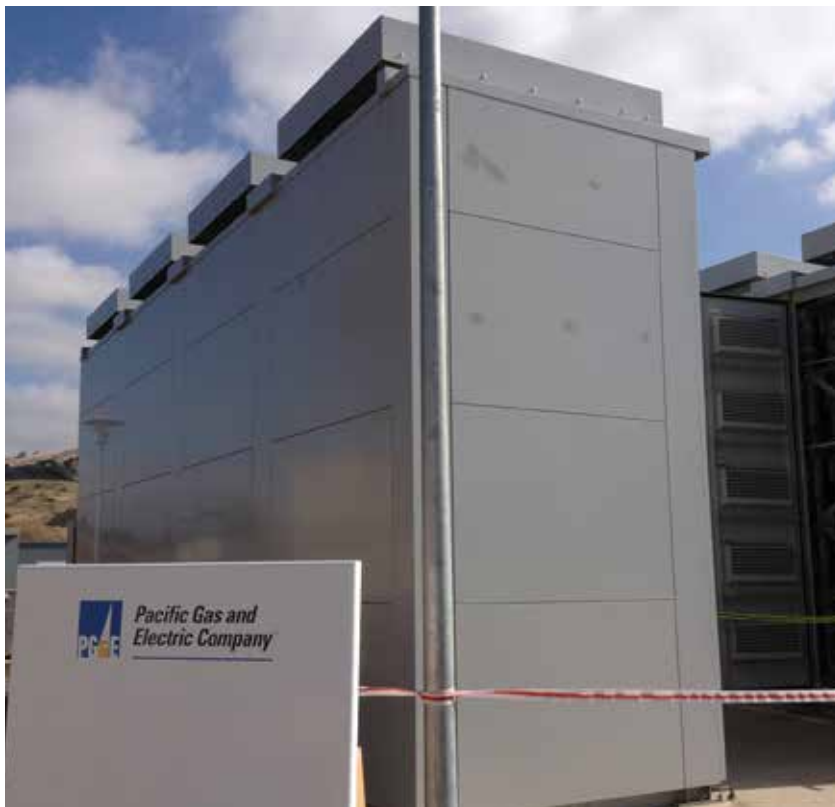
The Yerba Buena battery energy storage system (4-MW/28-MWH) is deployed at the end of a PG&E distribution feeder in San Jose, CA.
